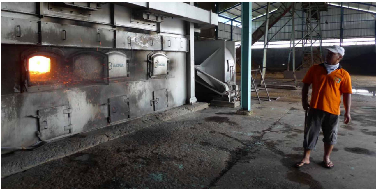
Figure 8.1: Boiler in a palm oil mill, using processing residues
